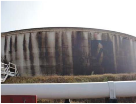
Figure 5. Tank T-6020 with spilled oil. El Maule earthquake 2010.
