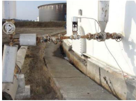
Figure 6. Tank T-6030. With tilt due to liquefaction soil lateral spreading. 2010 El Maule earthquake.
