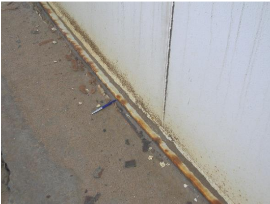
Figure 3. Horizontal sliding (80mm) Tank TK-201. 2007 Tocopilla earthquake.
