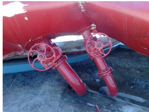
Figure 8. El Maule 2010, Chile earthquake. Large deformations of water pipes connected to shell tank, Santiago Airport.
