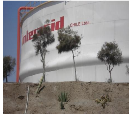
Figure 6. Tocopilla, Chile 2007 earthquake, sulfuric acid plant. Buckling of shell.
